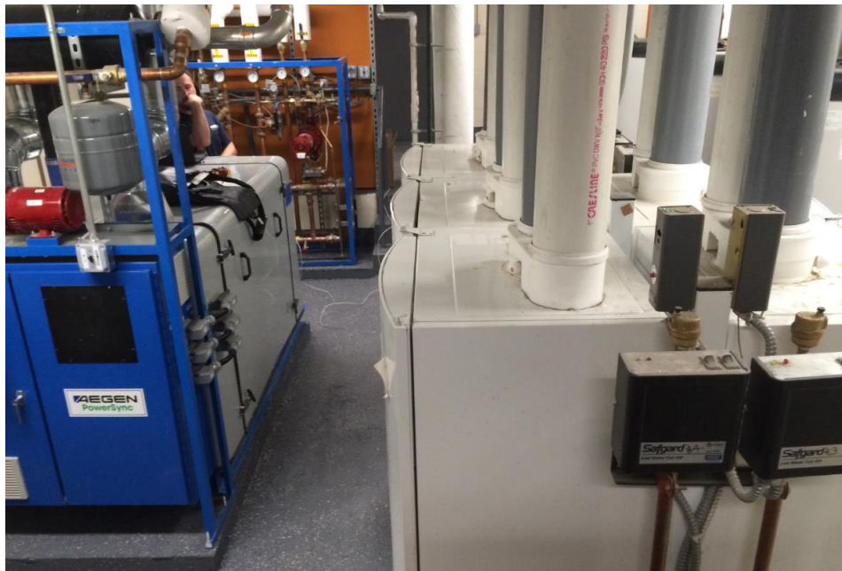
Picture #2: Boiler room, variable speed pumping, boilers, and CHP
