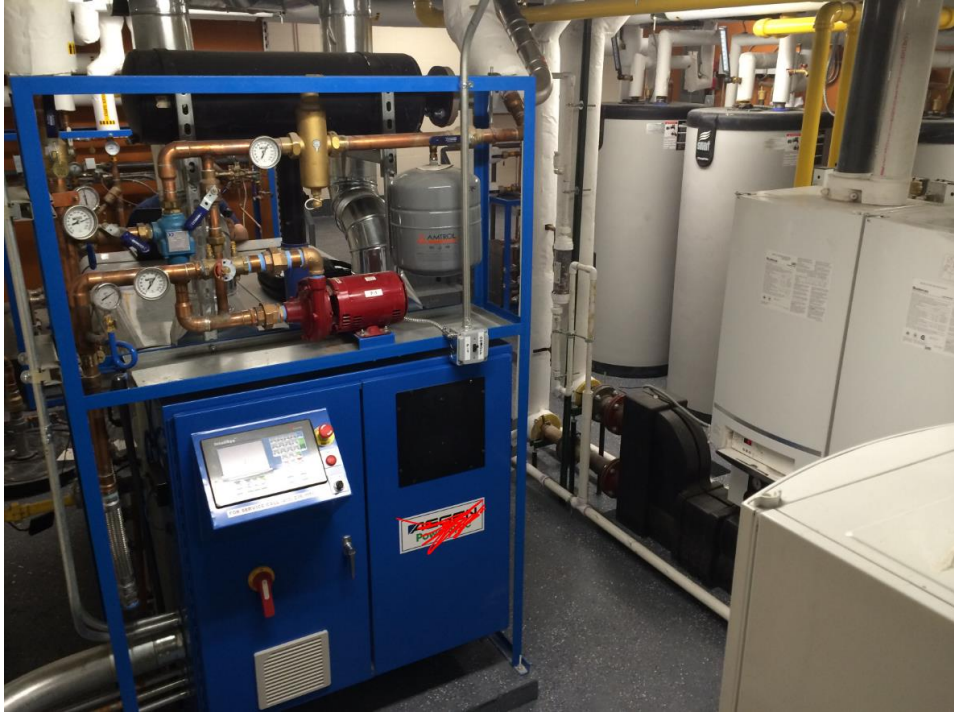
Picture shows the new CHP, High efficiency boilers, and water tanks
