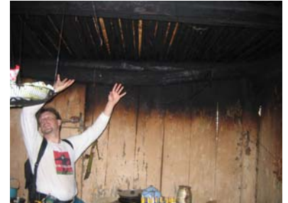
Martin discusses the project. The soot on the ceiling is obvious and between the cracks are the stalks of corn are visible.
